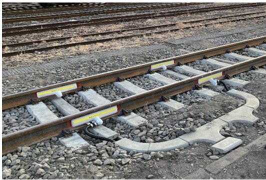
図5 輪重測定装置(ひずみゲージ部) Sensor for wheel load measuring device
